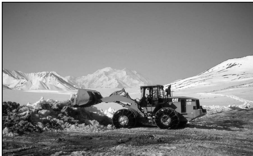
Large equipment is often required to open the 90-mile-long Denali Park road every spring, as shown in this photo taken near Stony Creek. photo courtesy of Sue Deyoe
